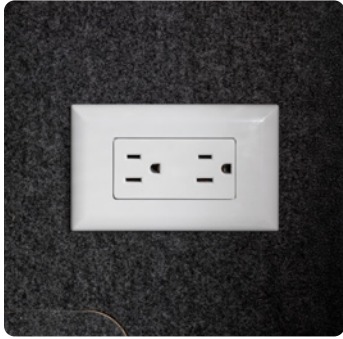
120-V Receptacle Located in Gear Garage (Rear Twin Bed)
