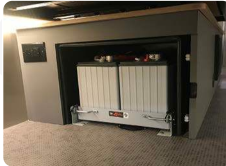
Battery slide-out drawers, locked. Two batteries shown.
